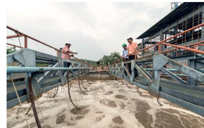
The effluent treatment plant at Lote.
