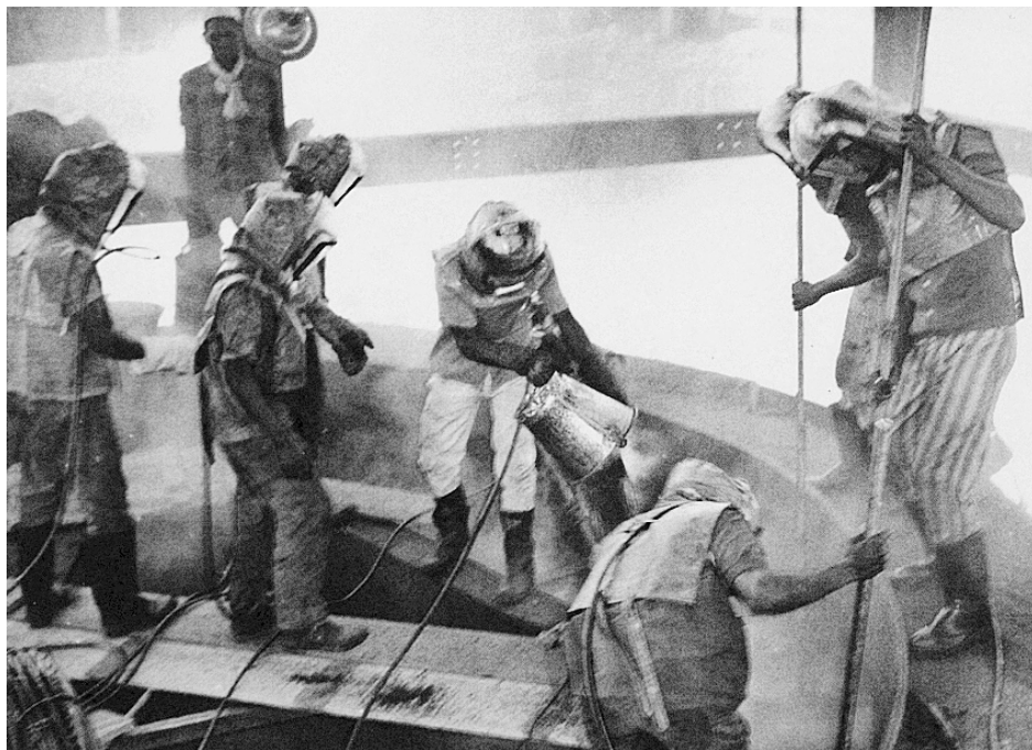
Part of the furnace being built. The outer shell under fabrication with buckets of fuming carbon paste being poured into the making of the side walls.
