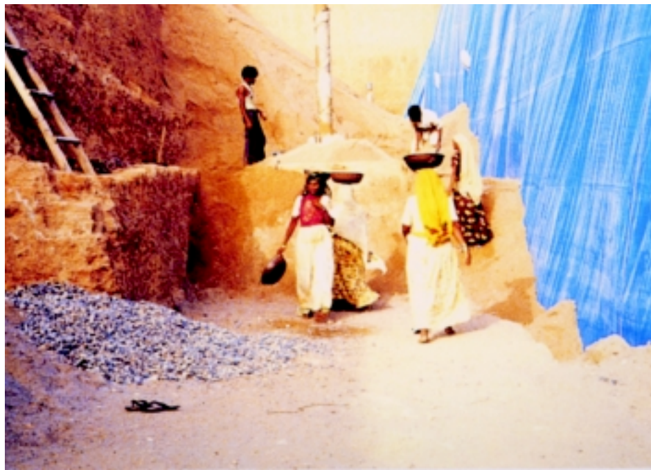
An underground dyke being built by Shri Vivekananda Research & Training Institute, Mandvi, which has done pioneering work for tackling the problem of water shortage in Kutch by recharging underground aquifers.
